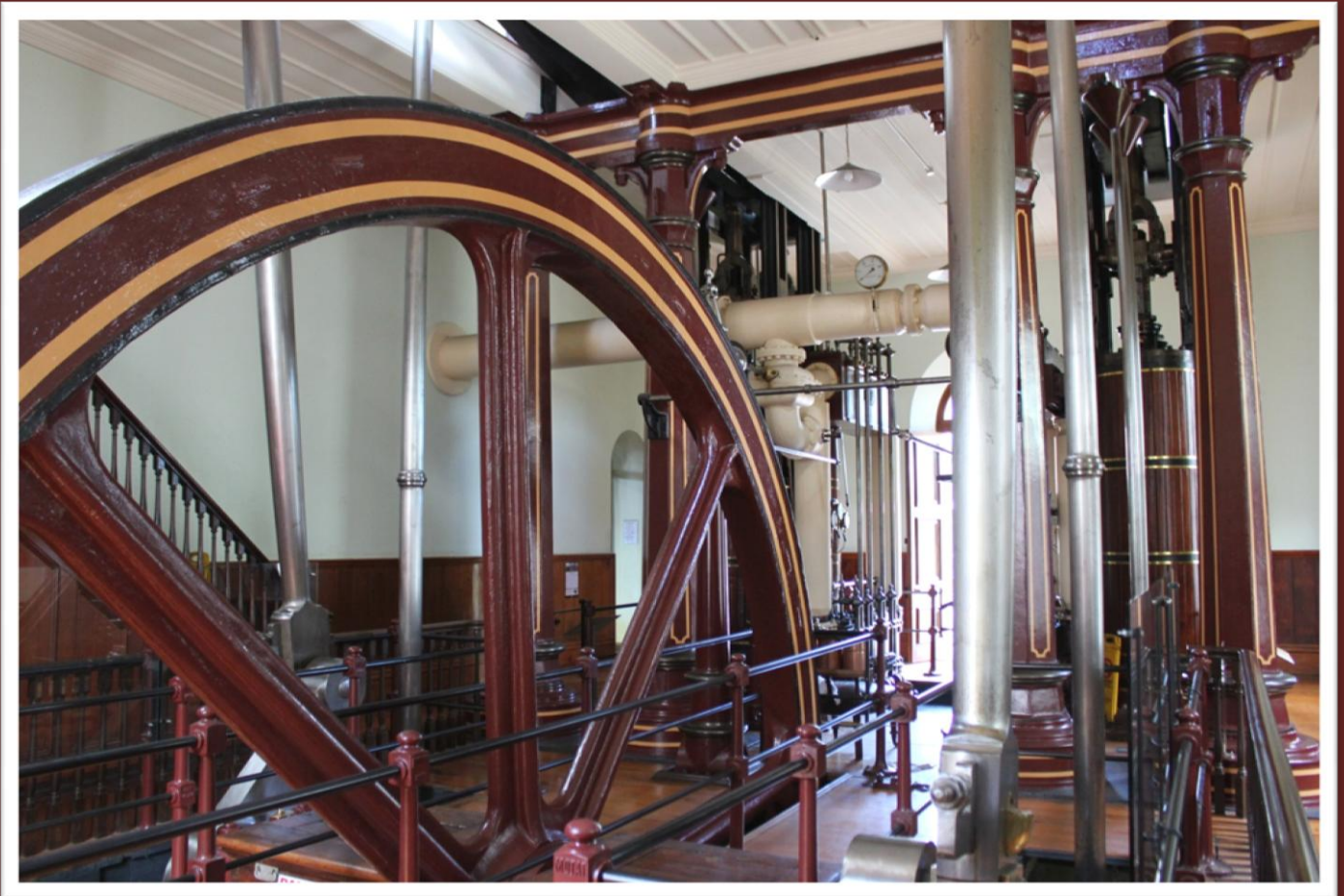
The 1877 beam engine at the former Auckland Waterworks and Pumping Station at MOTAT, Western Springs.
